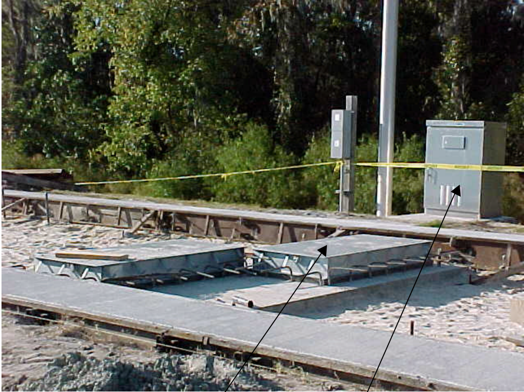
WIM Platform WIM Controller Enclosure Figure 2: Typical Type III WIM Scale
